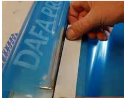
Remove one part of the liner and fix securely to the foil where the break is.
